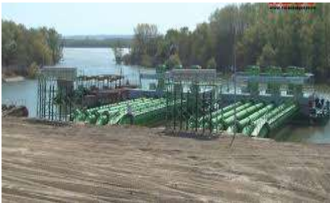
Figure 1. Pumping Station That Takes Water from the Danube
