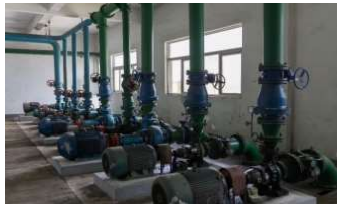
Figure 2. Irrigation Pumping Station
