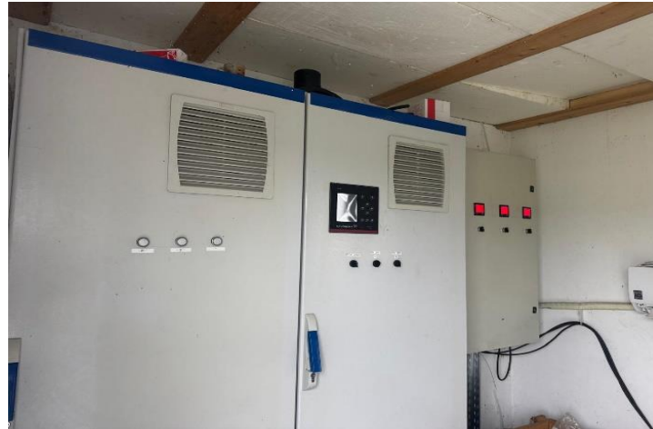
Figure 2. Electrical pump starting and control system of the existing pumping station, illustrating the conventional configuration used before the implementation of energy-efficient automation and frequency control.
