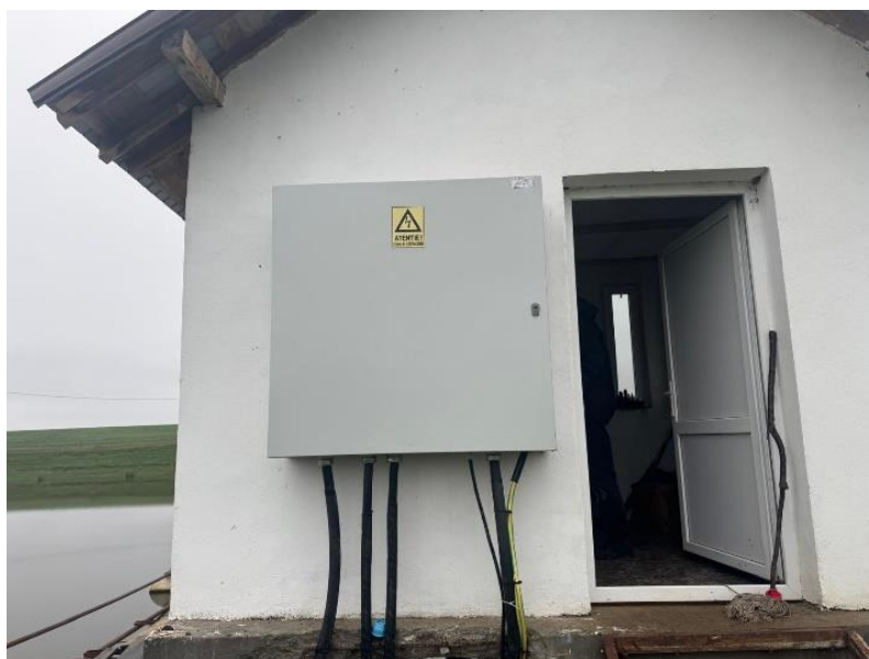
Figure 1. General view of the irrigation pumping station supplying the analyzed agricultural area, highlighting the arrangement of pumping units and the main hydraulic components prior to rehabilitation.
